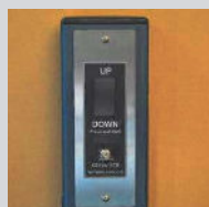
Key Switched Controls
